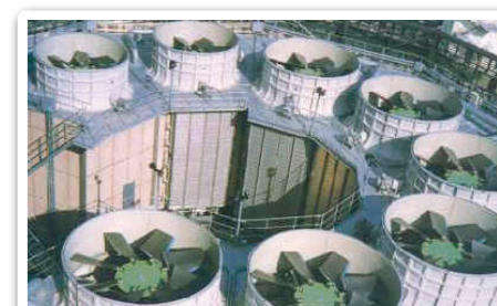
• Cooling Tower / Air Fin Cooler
